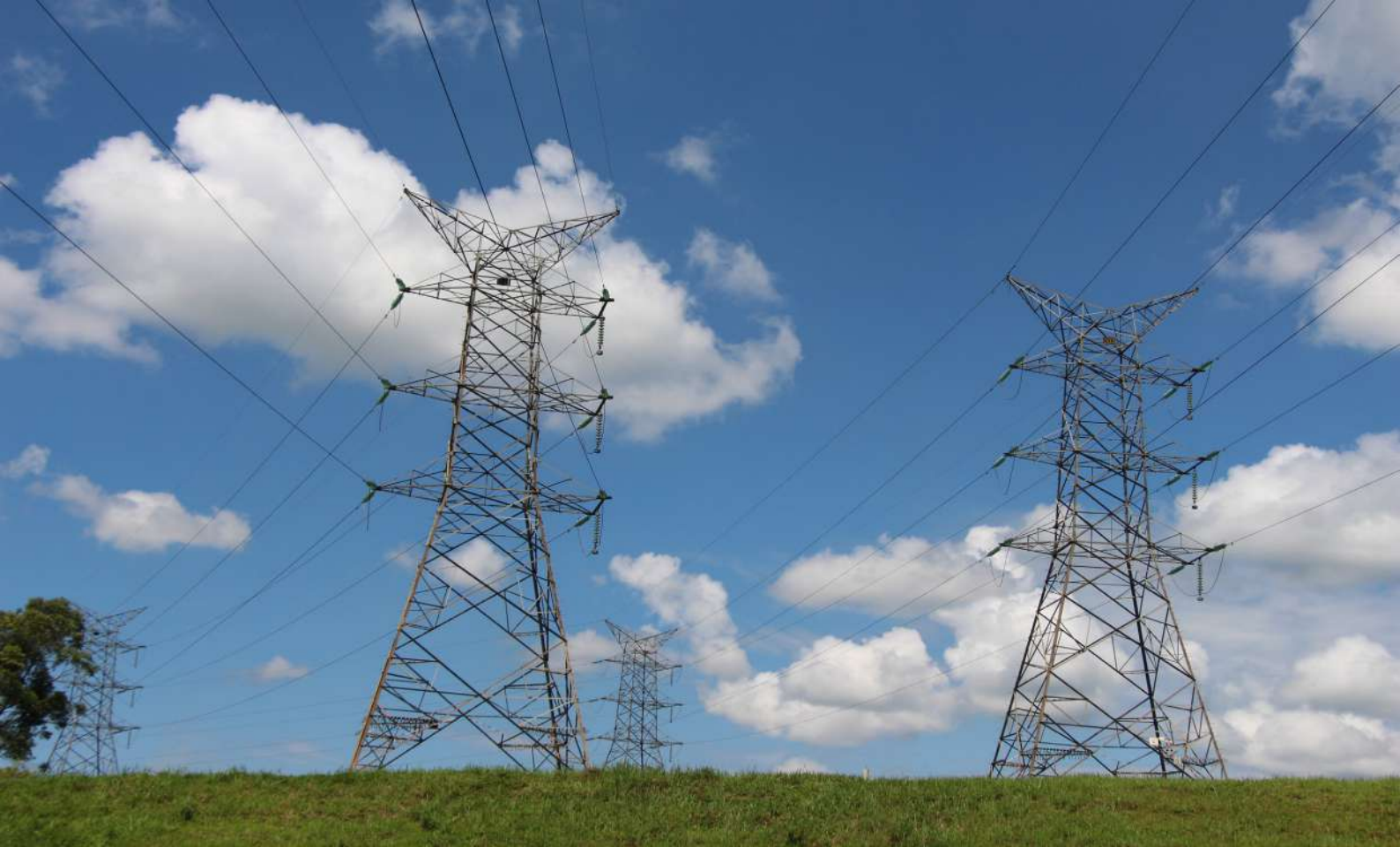
NELSAP IS WORKING ON A NUMBER OF TRANSMISSION LINES INTERCONNECTING THE NEL COUNTRIES
