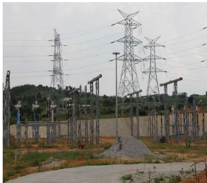
NELSAP will supervise construction of power Substations in Ngozi and Gitega (Burundi) for Euro 6.79M AfDB funding. The project is currently under appraisal
