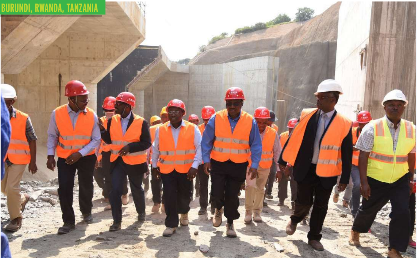
HON. COME MANIRAKIZA THE BURUNDI MINISTER FOR HYDRAULIC, ENERGY AND MINES, HON. AMB. CLAVER GATETE THE RWANDA MINISTER OF INFRASTRUCTURE, AND HON.DR. MEDARD KALEMANI THE TANZANIA MINISTER FOR ENERGY, VISIT THE SITE OF THE ONGOING CONSTRUCTION OF THE REGIONAL RUSUMO FALLS HYDROELECTRIC PROJECT (RRFHP)
