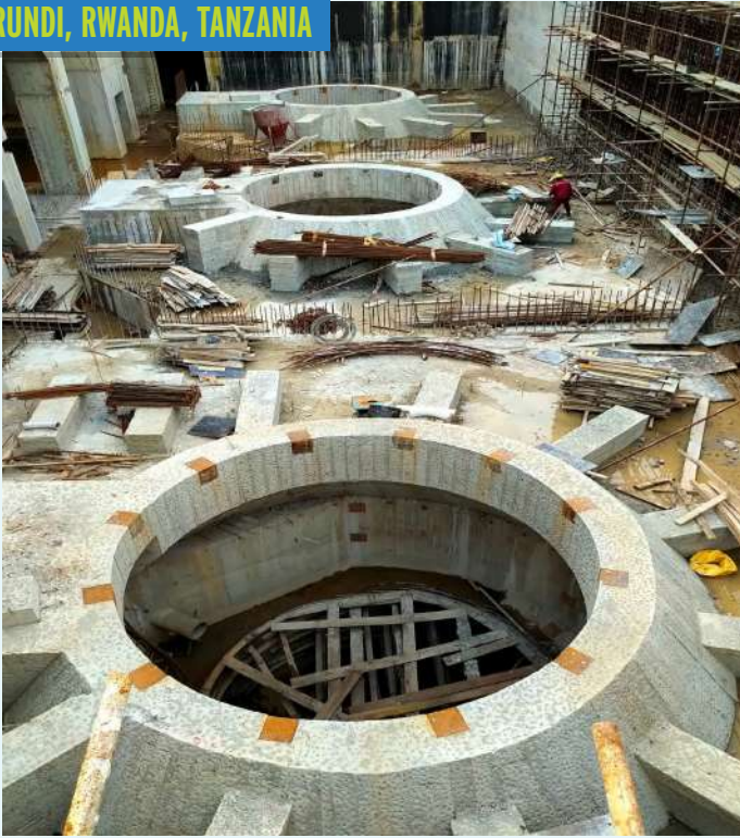
DRAFT TUBE AT THE POWERHOUSE
