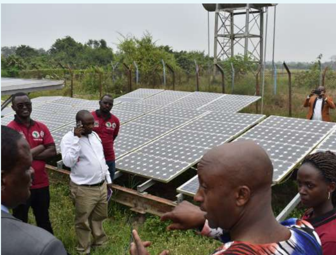
SOLAR WATER PUMP TO SUPPLY BOREHOLE WATER FOR HYGIENIC CLEANING AND PROCESSING OF FISH
