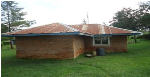
Wilson Shango James' House at Chesero Location: Kakamega County before the Project
