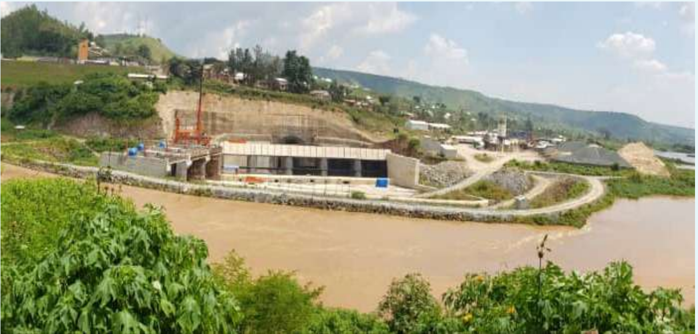
ONGOING CONSTRUCTION AT THE REGIONAL RUSUMO FALLS HYDROELECTRIC PROJECT (RRFHP) SITE. THIS PROJECT BEING MANAGED BY NELSAP-CU IS 61% COMPLETE AS OF FEBRUARY 2020
