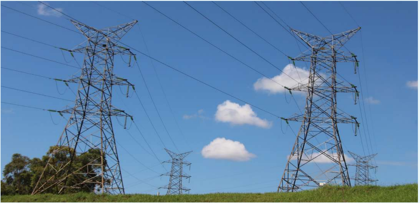
THE KENYA (LESSOS) - UGANDA (TORORO - BUJAGALI) OVERHEAD TRANSMISSION LINE. THIS IS ONE OF THE ONGOING PROJECTS UNDER INTERCONNECTION OF THE POWER GRIDS OF NEL COUNTRIES MANAGED BY NELSAP-CU
